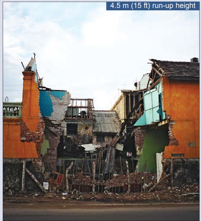
Damage to unreinforced masonry buildings within 100 m (330 ft) of the shore in Galle, near the reinforced concrete structures pictured on the left; wave run-up height in this area measured at 4.5 m (15 ft), destroying the structural integrity of the buildings
