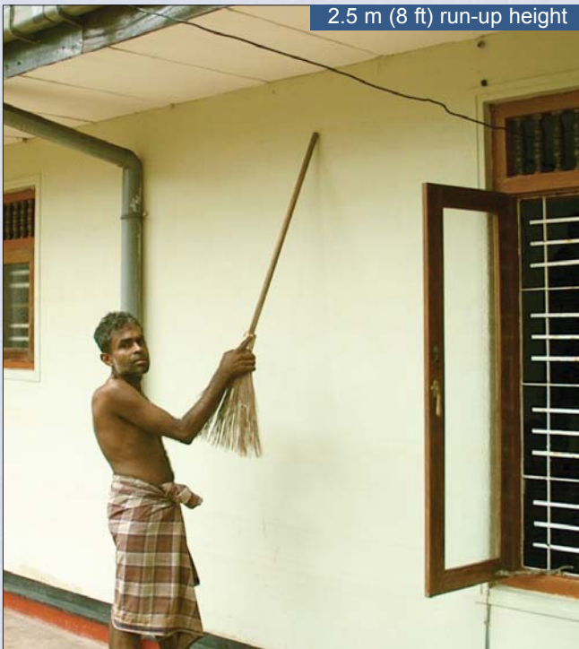
Single-story unreinforced masonry house located 170 m (560 ft) from the shoreline in Paiyagala village in Sri Lanka that was protected from the power of the waves by dense plantation and sustained only flood damage; a local resident indicates a water mark at approximately 2.5 m (8 ft)
