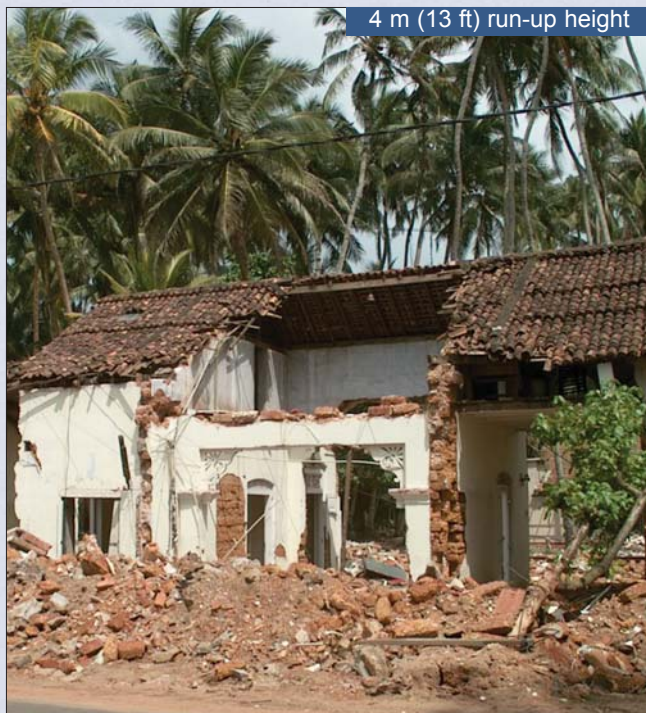
Typical damage to unreinforced masonry homes within 100 m (330 ft) of the coast in the village of Paiyagala in southwest Sri Lanka; run-up height at this location measured at 4 m (13 ft)
