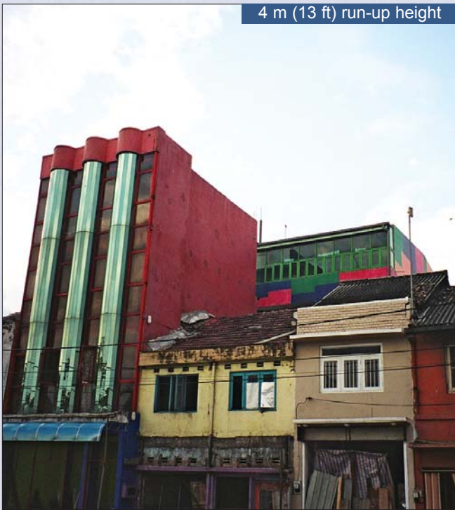
Damage to reinforced concrete commercial structures from wave run-up height of about 4 m (13 ft) within 100 m (330 ft) of the shore in the city of Galle in southern Sri Lanka; structural damage was limited to the ground floors of these structures (note undamaged curtain wall panels above the ground floor level)
