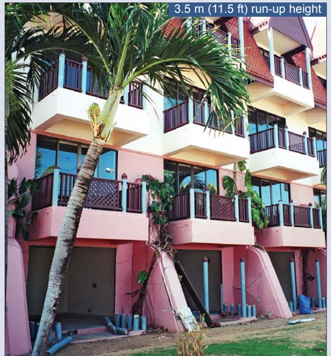
Damage from run-up heights between 3 and 3.5 m (10 to 11 ft) to a reinforced concrete hotel 100 m (330 ft) from the coastline on Phuket Island, Thailand; since contents and non-structural damage was limited to the ground floor, clean up operations were completed by the time this photo was taken just one month after the event
