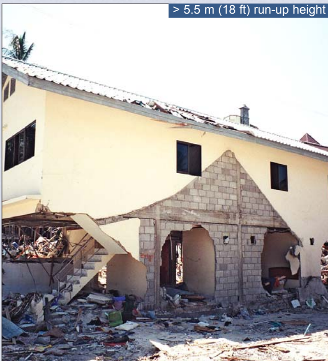
Damage to a two-story reinforced concrete structure located 200 m (660 ft) from the northern shore of Phi Phi Island in Thailand, where wave run-up height exceeded 5.5 m (18 ft) above the foundation
